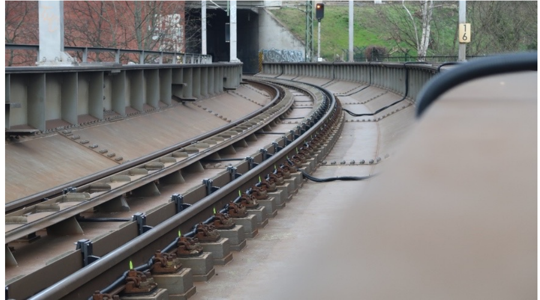
Magnetic inductive sensors at the elevated rail of a bridge (1.2m spacing).
