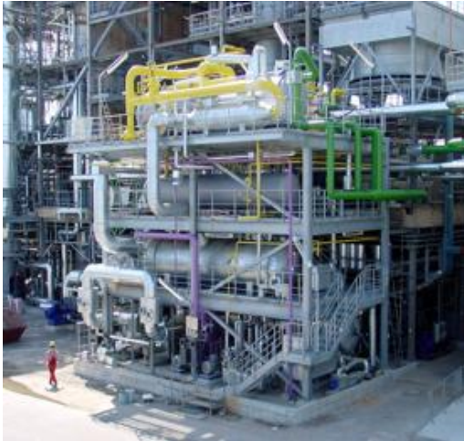
Industrial absorption machinery (1.6 MW cooling capacity at -30°C) as part of a chemical plant, Germany.
