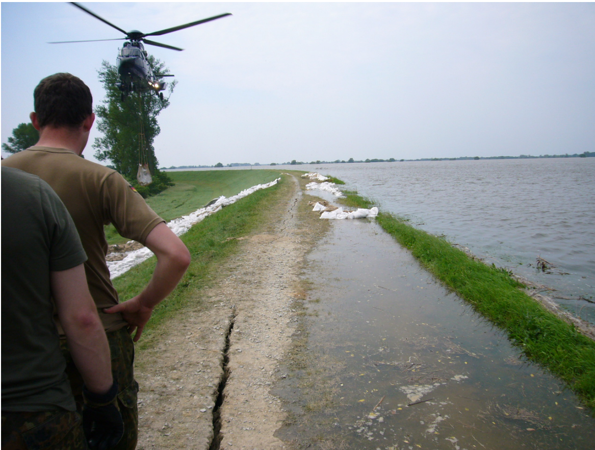
Figure 1: Dike at the river Elbe close to Fischbeck on June, 9 – 10 hours before the break (Ellmann, 2013)
